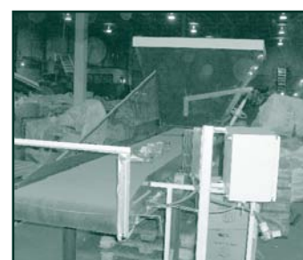
Containers on conveyor belt pass through presence sensing device to be counted
